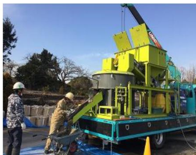
▲ Vehicle-mounted manufacturing plant (Mobacon)
